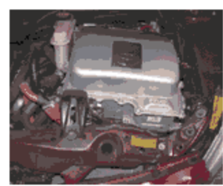
The inverter/converter assembly in this Prius is located at the top of the engine compartment near the radiator support, making it susceptible to damage in the event of a front-end impact such as this.
