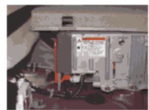
When you remove the spare tire cover and necessary interior trim panels behind the back seat of the Prius, you can access the service plug and disconnect the high-voltage battery pack from the system.
