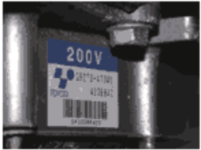
Note that the label on the inverter/converter of this Prius rates the high-voltage system at 200 volts, which is more than enough to kill you instantly.
